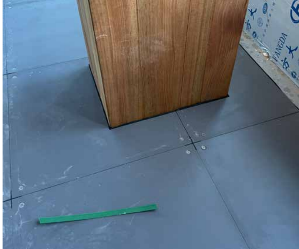
Raised Access Floor
